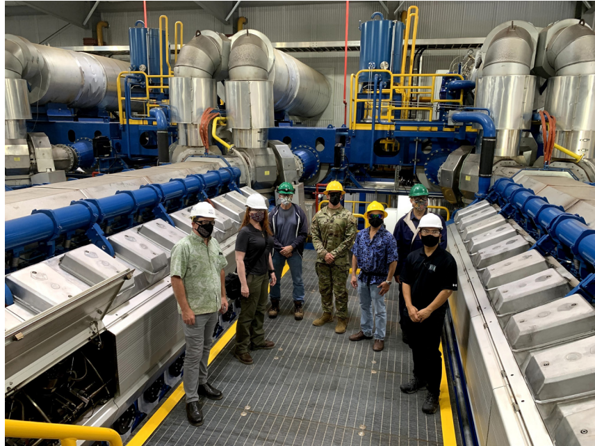
Figure 33. inside the biofuel power generation plant at Schofield Barracks. Source: US Army
