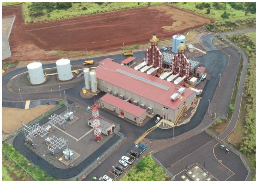
Figure 34. Aerial view of the Biofuel power generation plant at Schofield Barracks. Source: US Army
