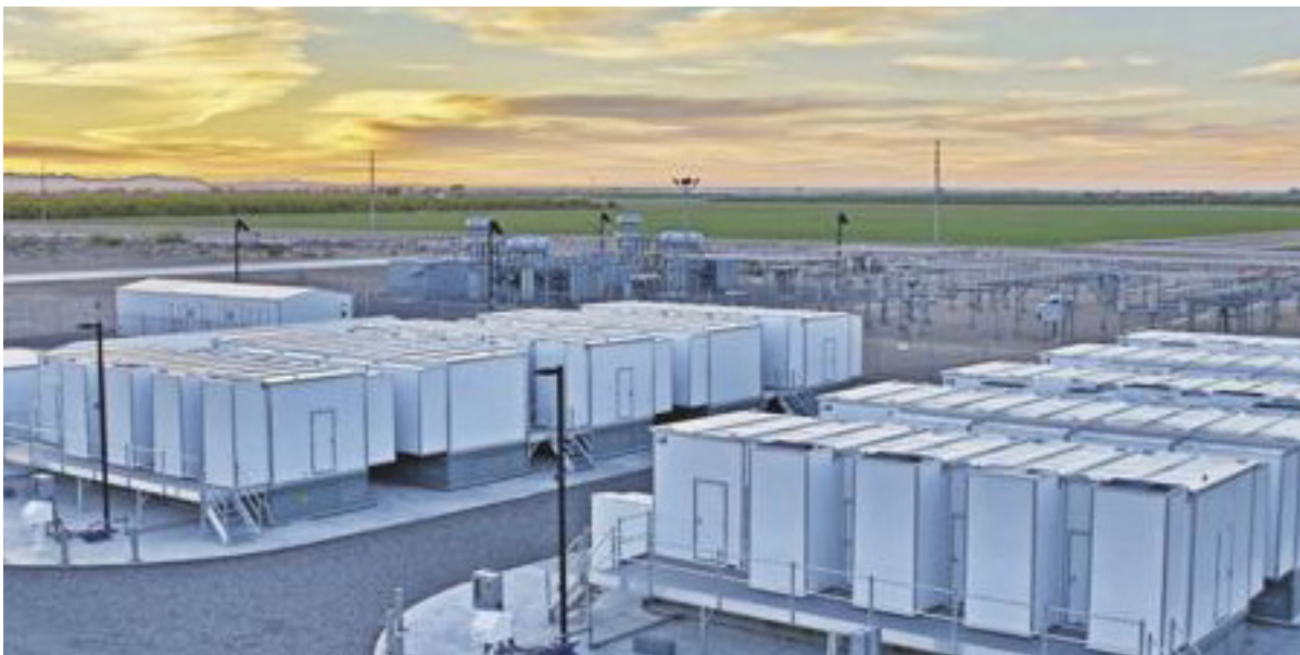
Figure 46. Microgrid in the Marine Corps Air Station (MCAS) in Yuma, Arizona. Source: www.eei.org
