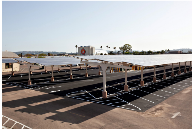
Figure 47. Carport soSolar cuitions in Miramar air station Car Source U.S. Marine Corps
