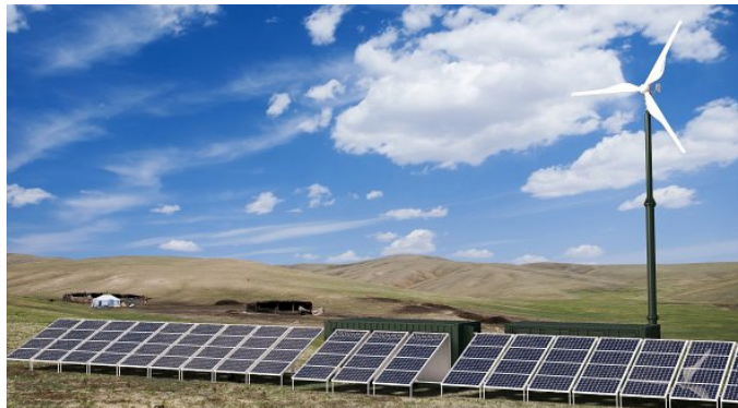
Figure 16. Hybrid Power Generation and Management System
